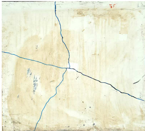
Fig. 11 The dynamic-static crack pattern of the slab T8F
