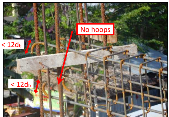
Fig. 24 Typical deficiencies in exterior beam-column joint
