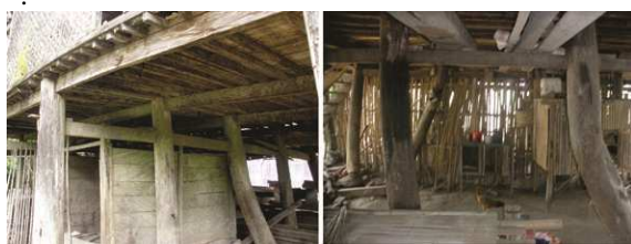
Fig. 1. Bent column in center position
