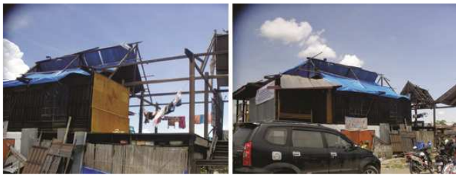
Fig. 6. The wind destroyed part of the wall
