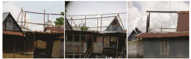
Fig. 4. Roof sheet flew with the wind
