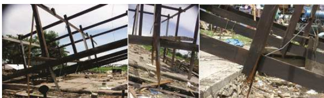
Fig. 8. The lower column group has been broken due to the wind.
