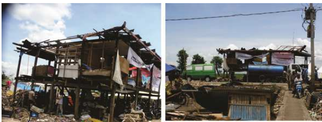
Fig. 7. Wall and roof structures destroyed by the wind.
