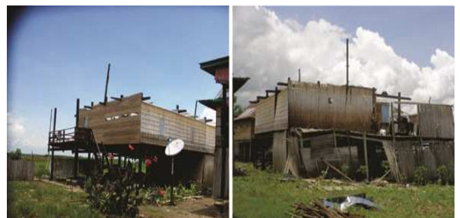
Fig. 5. The roof structure destroyed by the wind
