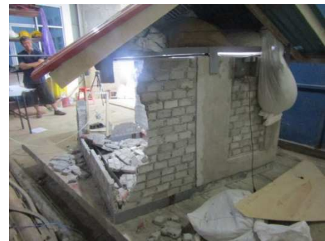
b. Condition of the Back of the Specimen
