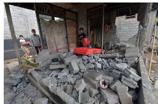
Fig. 1 Damage Simple Residential Houses Due to Earthquake
