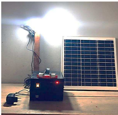
Fig. 10 Illuminated lighting bulbs with the developed system under operation
