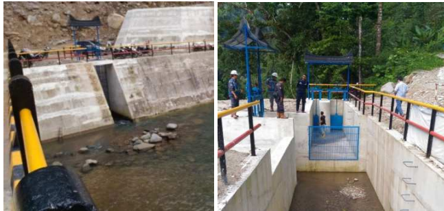
Fig. 2 Intake and Settling Tub
