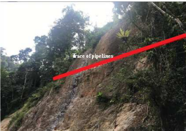
Fig. 4 Pipe Network Conditions on Slopes
