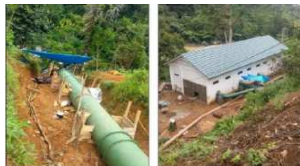
Fig. 1 Penstock and Turbine House,
