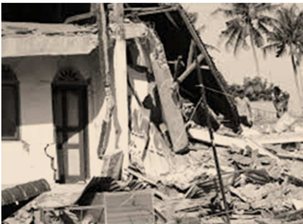
Fig. 3 Samples of two houses constructed of reinforced concrete with rigid frame joints which collapsed during the Pidie Jaya earthquake
