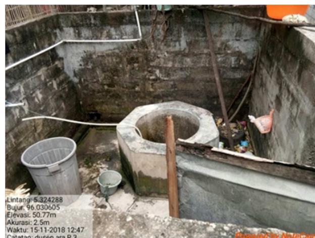
Fig. 14 The condition of sanitation, No WC.
